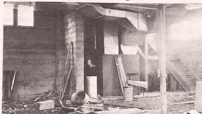
Boy, did that furnace make a difference. For several Sundays heat had been supplied by a flame in an oil barrel in the basement and the heat coming through holes in the floor.
