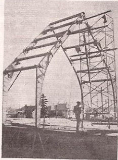
Two archs are up. The most difficult period past. These archs, the first of this kind used in Calgary, had been ordered and were on the way to St. Mark's, and the church had no money. But the prayers of this church family were heard. From here on it seems till the church was completed, things went on very well. Thanks to all, from the contractor to the water boy.
